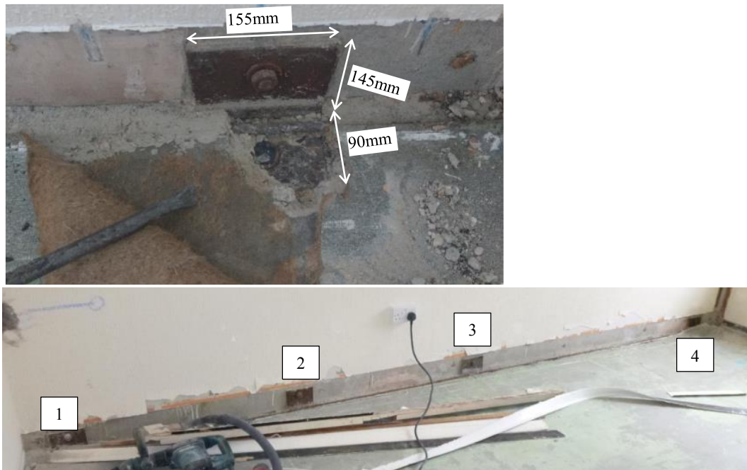
Figure 12 Bromyard House – L-brackets were found along the length of the cross-walls (location 8)
