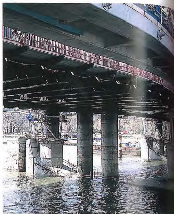
Above The slip-impact beams are just visible at low tide. The concrete at each end of them will be removed once the deck installation is complete.
