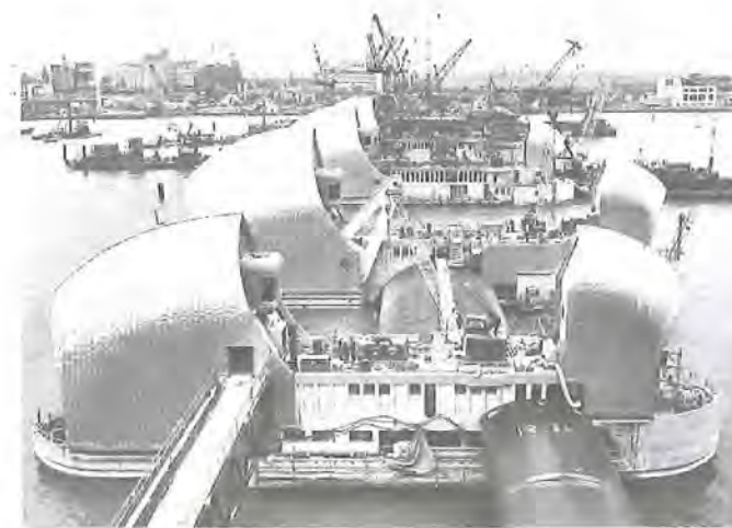
Far left: up-river view of the piers clad in stainless steel on laminated timber frames to protect the operating machinery. The concrete has been detailed to disguise waterline staining. Reminiscent of Sydney Opera House, the shells are being fixed in place by Tysons of Liverpool.
