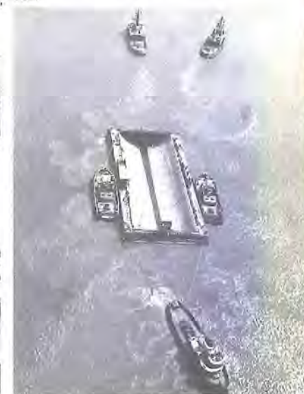
Below: a 61 metre span cill being towed into position between the piers before lowering to the river bed.
