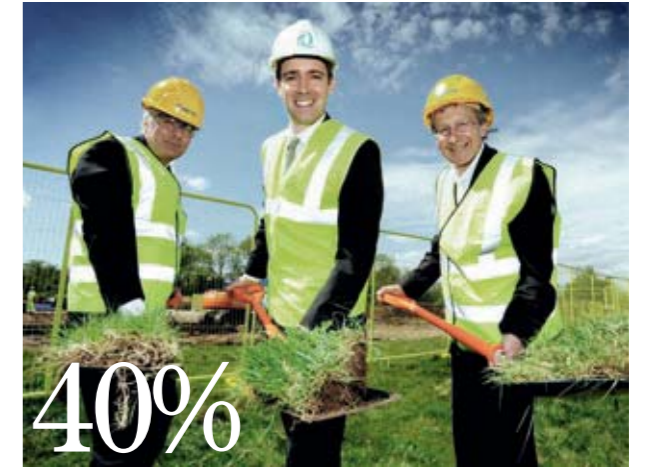
Breaking ground in Oxford Our development partnership with Oxford City Council started work on site this year. Barton Park will provide 885 much needed new homes for Oxford, 40% of which will be affordable.
