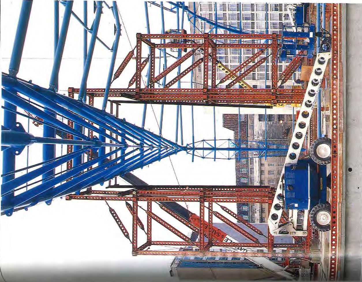
Temporary steel falsework locates and supports the arch sections after they have been craned into place.
