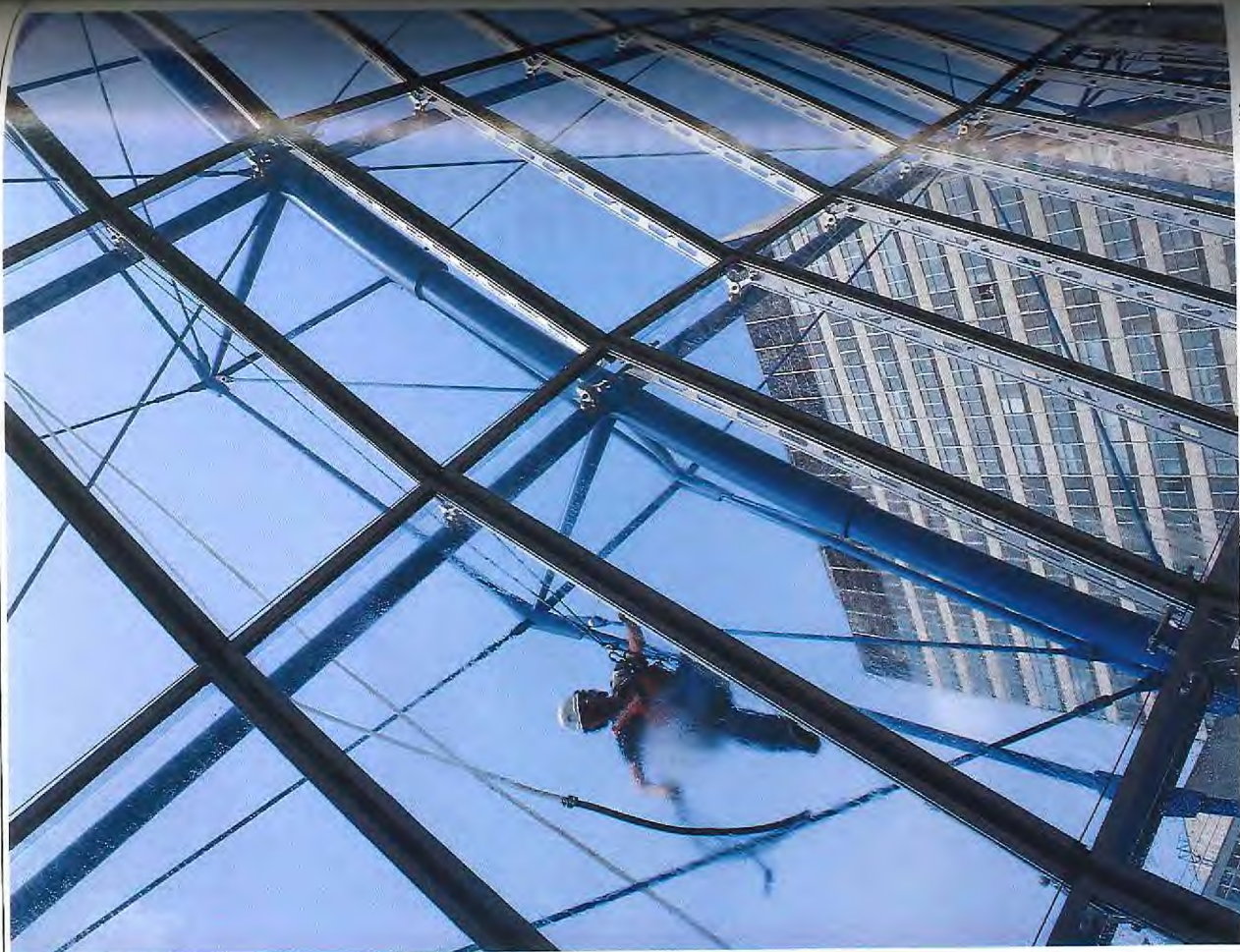
A workman tests the seals on the roof glazing. The prismatic bow-string truss construction is visible.
