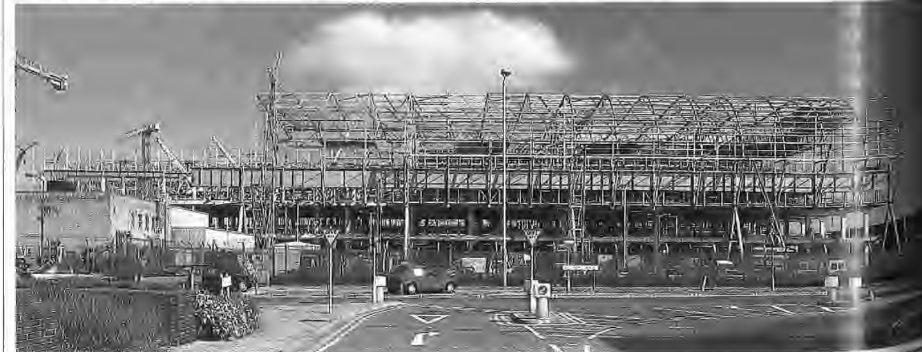
NOW, VOYAGER: Structural steelwork is well under way on British Airways' £150m World Cargo Centre at Heathrow Airport in west London. Work on the project, which is being project managed by British Airways Property, started
