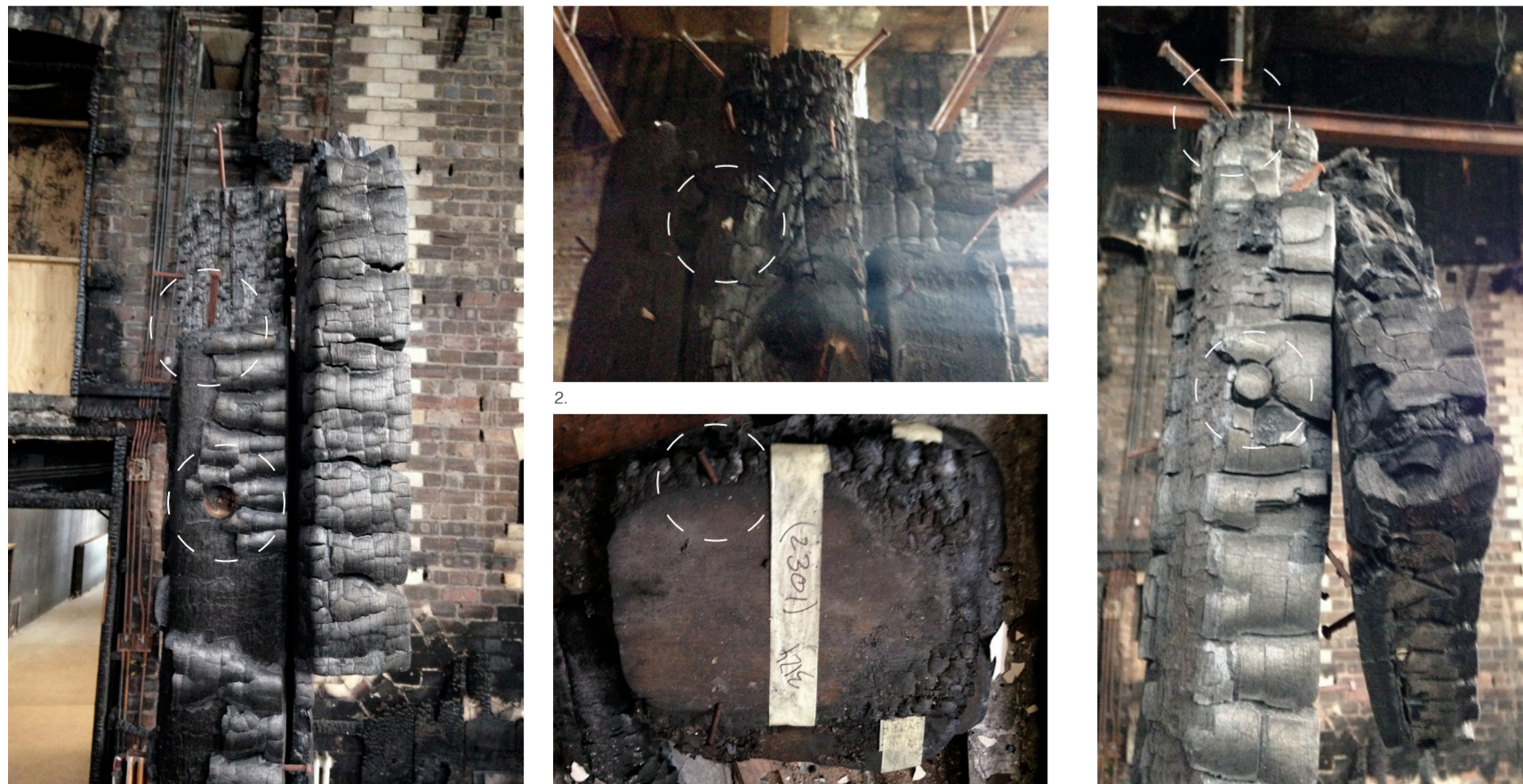
1. Side elevation of the lower post and timber plate. 2. Outer elevation of the lower post. Nails outer fascia highlighted. 3. Back elevation on timber plate. Screws driven with an angle securing the plate highlighted. 4. Side elevation of the lower post. Timber dowel and nail securing the upper post highlighted.
