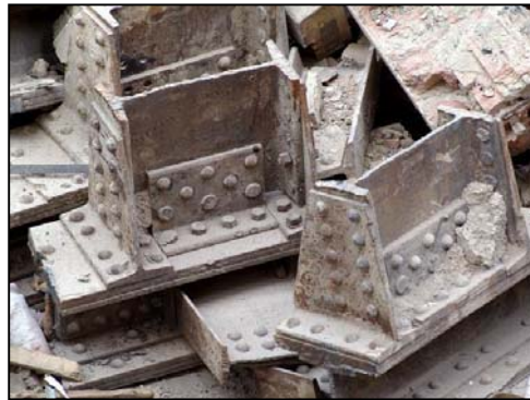
Segregated steelwork from the demolition of Unilever House (main building) prior to recycling
