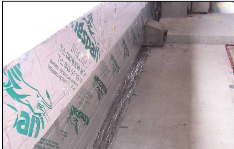
Figure 2 - Kingspan Insulation used to close gap between floorslab and wall.
